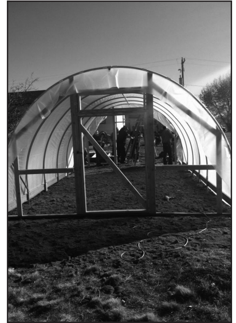
A hoop house, or greenhouse, being built on the Duck Valley reservation.
