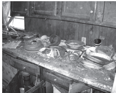
Ms. Debra's kitchen—cleared and gutted by Appalachian State University and St. Augustine's College volunteers—is ready for rebuilding when the government gives the green light.
