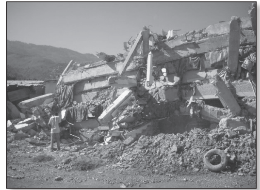
A man examines the damage of a Port-au-Prince school building following the January 12 earthquake.
