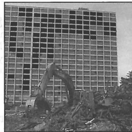
Demolition proceeds at Chicago's Cabrini-Green public housing project, as the city and housing authority tear down low-income high-rise housing to make way for lower density low- and mixed-income developments. (Photo by Peter Schaugnessy, Policy Research Action Group)
